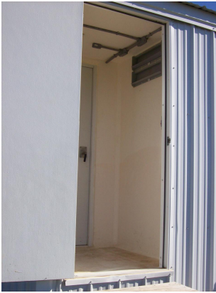
A view of the baffle inlet in the chamber
