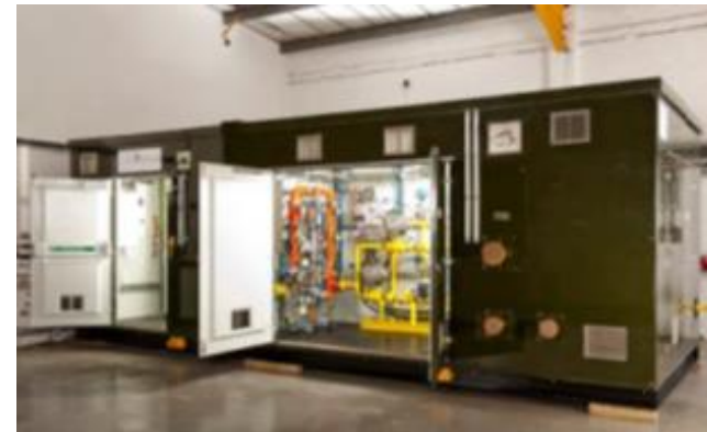
Biomethane Network Entry Facility
