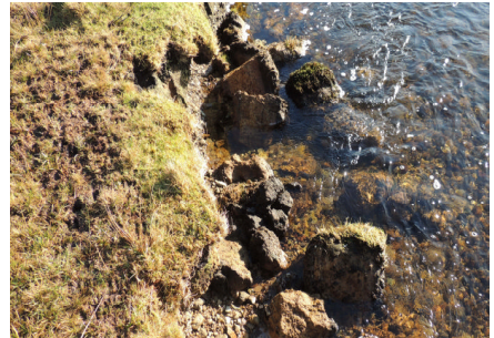
Figure 3. Eroding channel bank and poaching damage in FPM catchment
