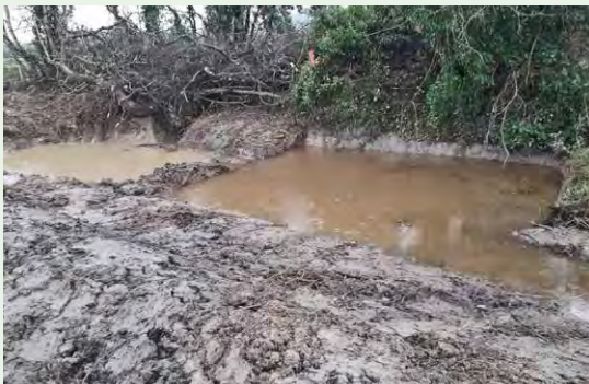
Figure 5. A two chamber settlement pond installed down drain in a fast flowing eroding farm connection drain to prevent sediment run-off to the river Allow (source Michael Morrissey IRD Duhallow Farming for Blue Dot Catchments EIP Project March 2021).
