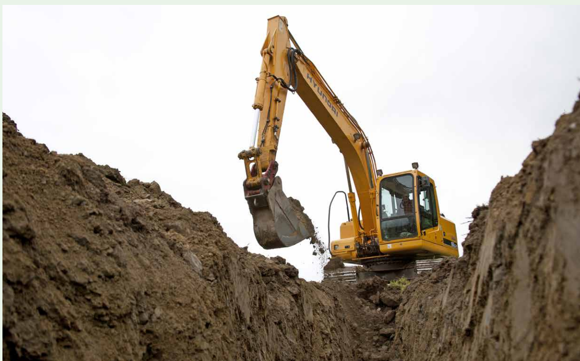
Figure 2. The drain depth will depend entirely on the depth of the impermeable layer.
