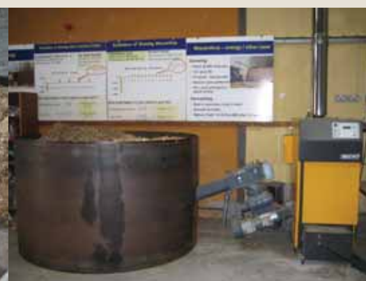
FIGURE 3: Willow chip combustion at Oak Park.
