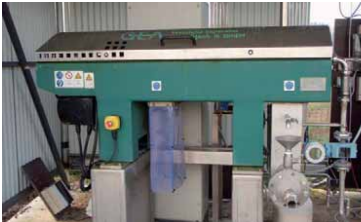
A decanting centrifuge installation used to separate pig manure at Moorepark.
