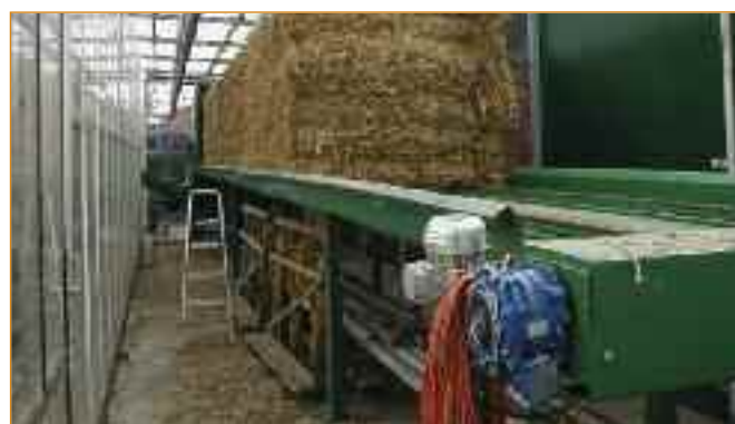
Straw bales being fed into shredder and combustion chamber.
