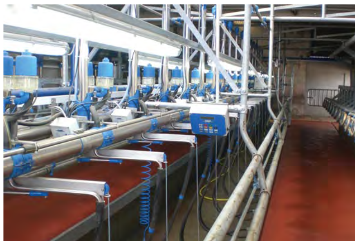
FIGURE 1: A well-lit parlour with two rows of double fluorescent fittings.
