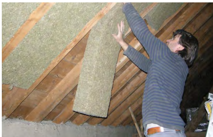
FIGURE 1: Installation of insulation boards made from grass fibre (Source: Stefan Grass; www.gramitech.ch ).
