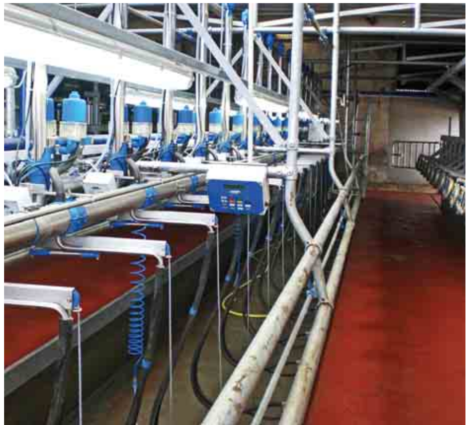
A well lit parlour with two rows of double fluorescent fittings.
