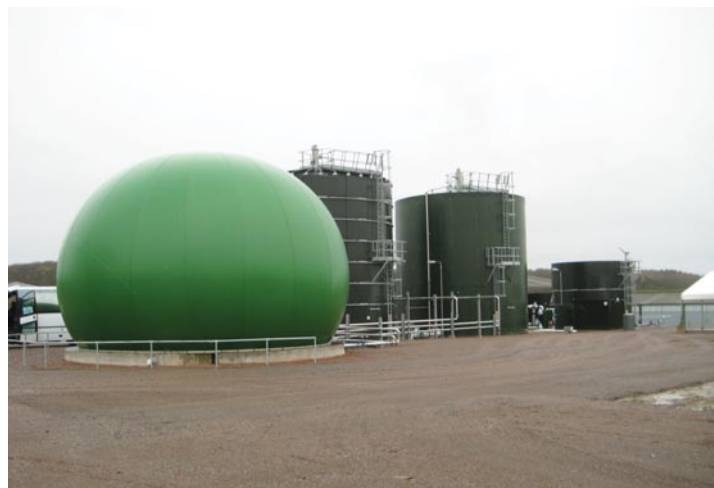
Anaerobic digester at the Agri-Food and Biosciences Institute, Hillsborough, Co Down.
