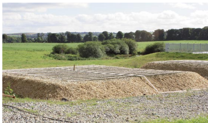
Woodchip filters used to treat soiled water for re-use to wash down yards.
