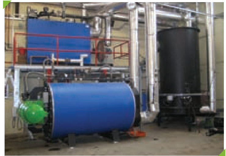
Figure 2: Biomass CHP plant at Oak Park featuring the gasifier (black cylinder on right), gas combustion chamber (blue cylinder in the centre) and the Stirling engine (green unit attached to the combustion chamber).
