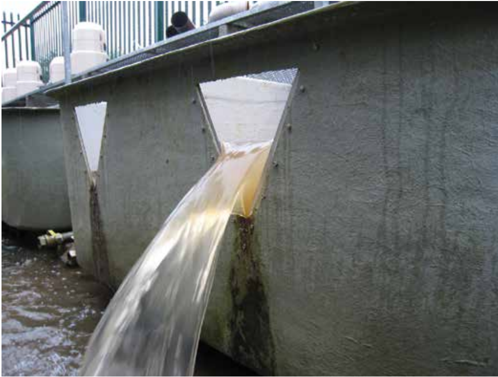
Figure 1. Tanks, V-notch weirs and automatic samplers installed at the bottom of grassland plots to monitor water volumes and nutrient losses in overland and subsurface drainage flow.
