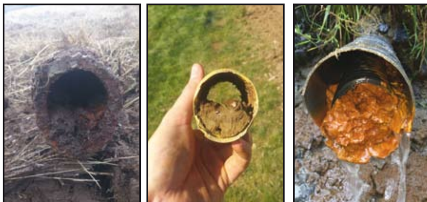
Figure 3. Examples of blockages in drainage pipes.
