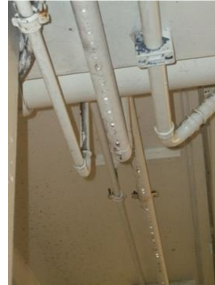
Dripping from ceiling
