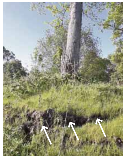
The recent cracks in the soil around this tree on a bank indicate it has already started to fail.
