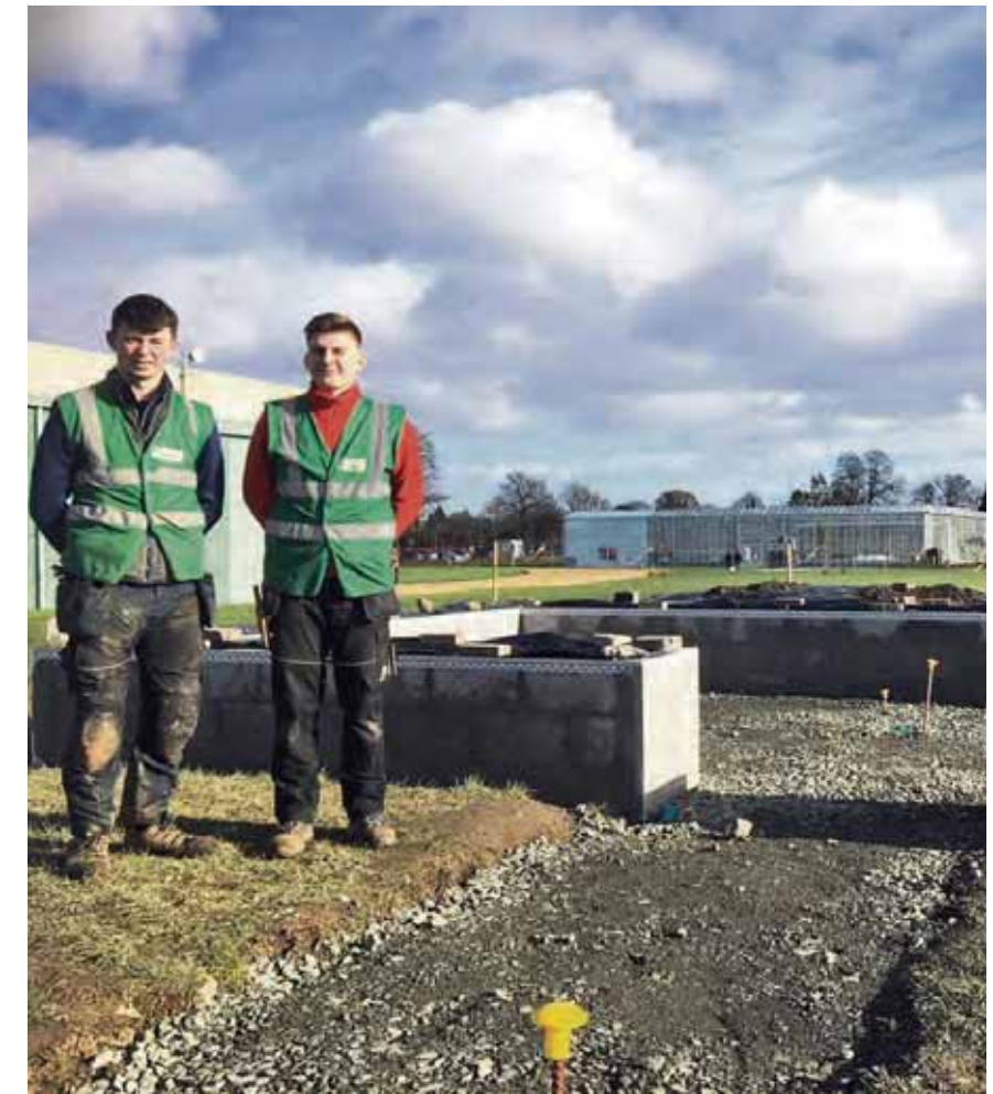
Zack Meehan and Bartek Wojcik pictured at the student garden building project which is under construction at the Teagasc campus in Ashtown Dublin 15.
