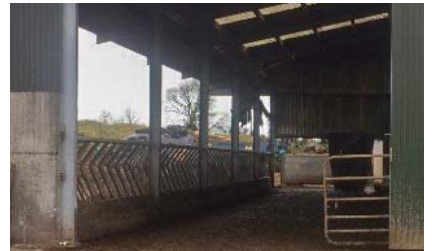
Protruding gates can cause injury to animals.
