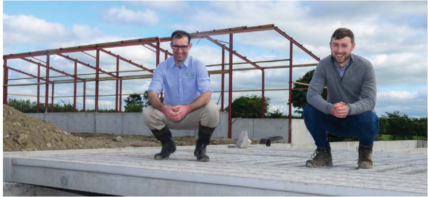
Teagasc advisor James Mimmagh and Eanna Galvin review construction work for the Galvins' new dairy facilities.
