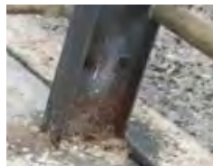
Stanchion showing corrosion. Painting the base of stanchions and cubicles will prolong their life.
