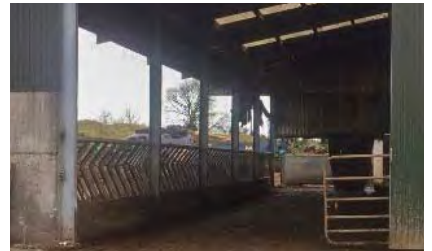
Protruding gates can cause injury to animals.
