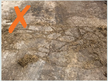
Cracks in silage base must be repaired before use to make it leak-proof.
