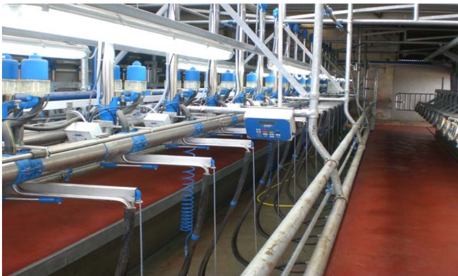
Figure 5: Well lit parlour with 2 rows of double fluorescent fittings
