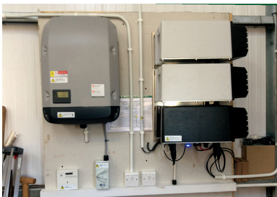
Battery storage enables you to save excess power generated.
