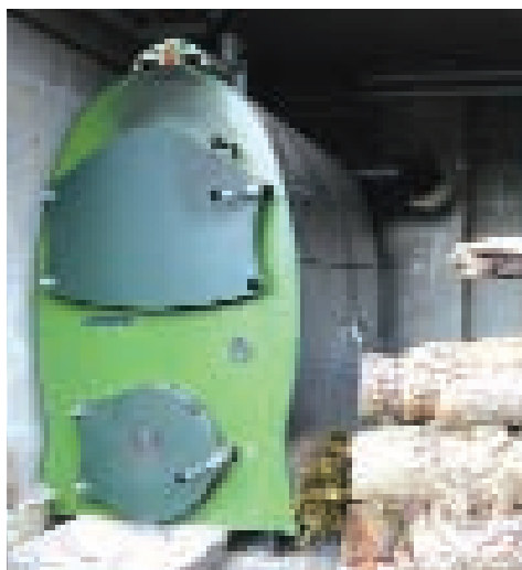
Wood log central heating boiler
