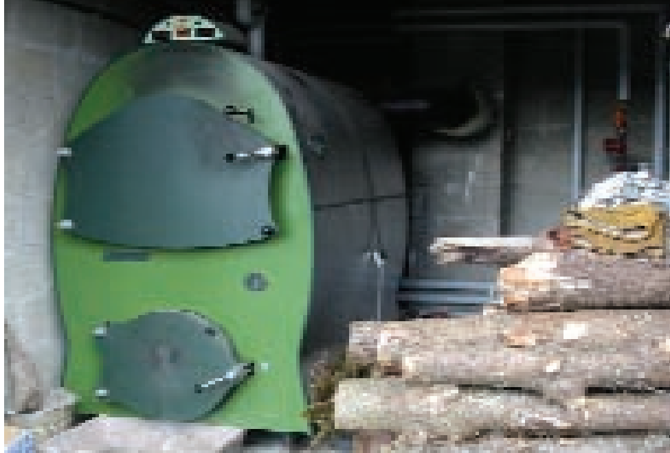
The Sustainable Land Use Company's log boiler
