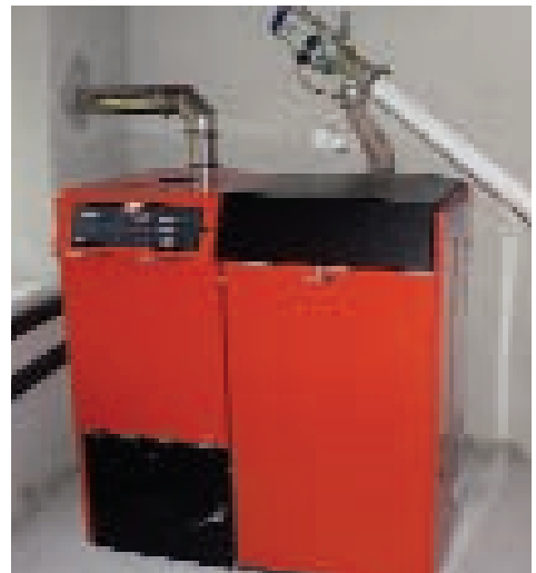
Wood pellet central heating boiler
