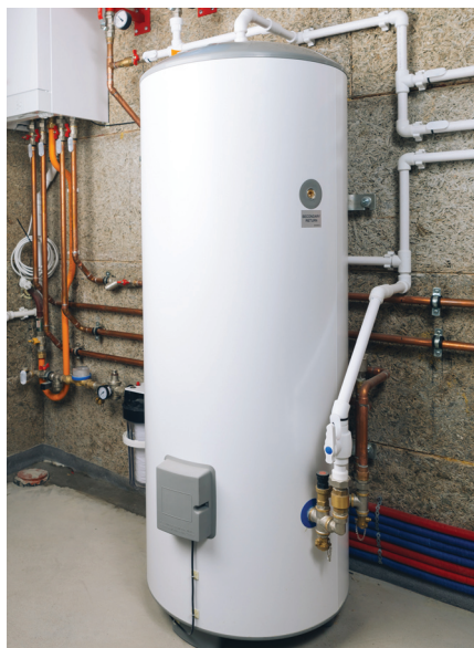
Hot water and heating can be supplied by heat pumps.
