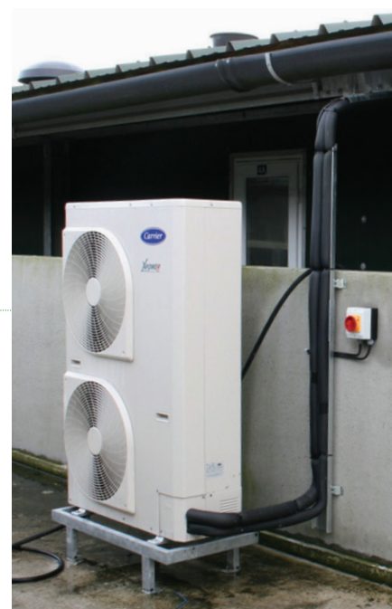
Heat pumps capture energy in the air, ground or water and deliver it to buildings.
